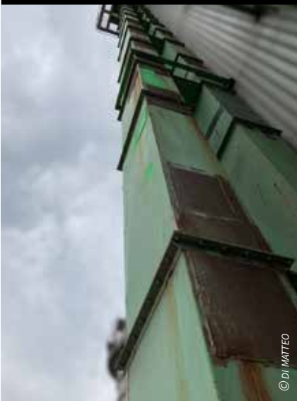
Figure 5: example of worn shaft casing that was repaired by patchwork
