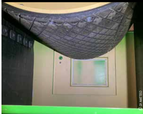
Figure 8: segmented drive pulley lining with large inspection door
