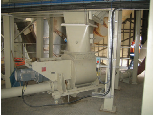
Fig. 4 (right): ODM – Injector gate IZS, for pneumatic feeding into the conveyor pipelines.
